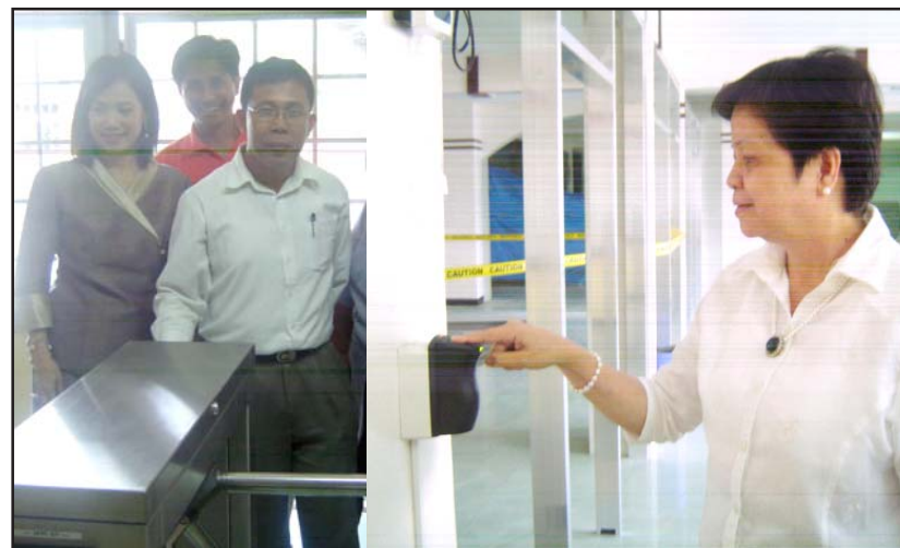
Dr. Fredie Bernal swipes his card at the access control system (left) while Dr. Isabel Inlayo, CHED IV-A Director tries out the biometrics time and attendance system (right).
